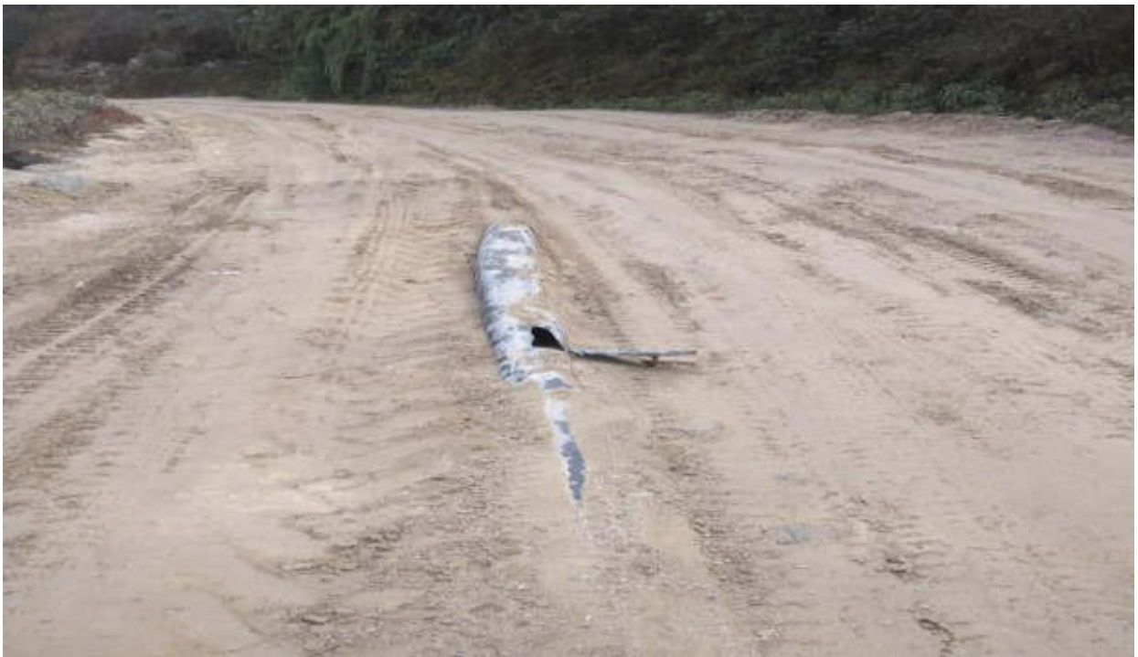
Damage of HDPE pipe at the middle of road, Khandbari
