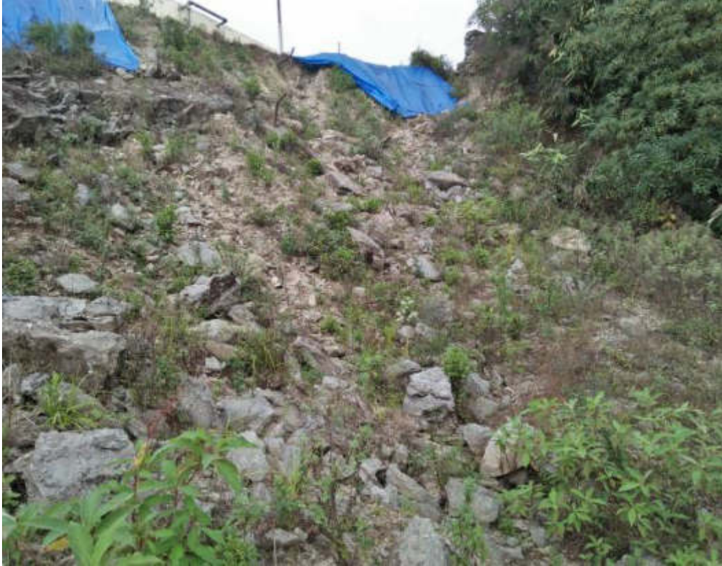
Landslide at D/S of Kuwapani WTP, Khandbari
