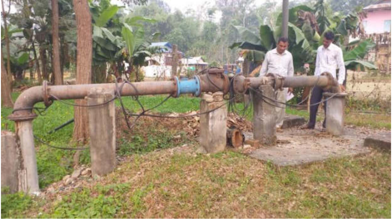
Outlet arrangement of Bore Hole Platform at Water Treatment plant, Belbari
