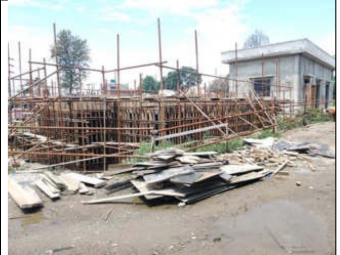
Figure: Poor Housekeeping but hard barricading done in Sallaghari site of TP02.
